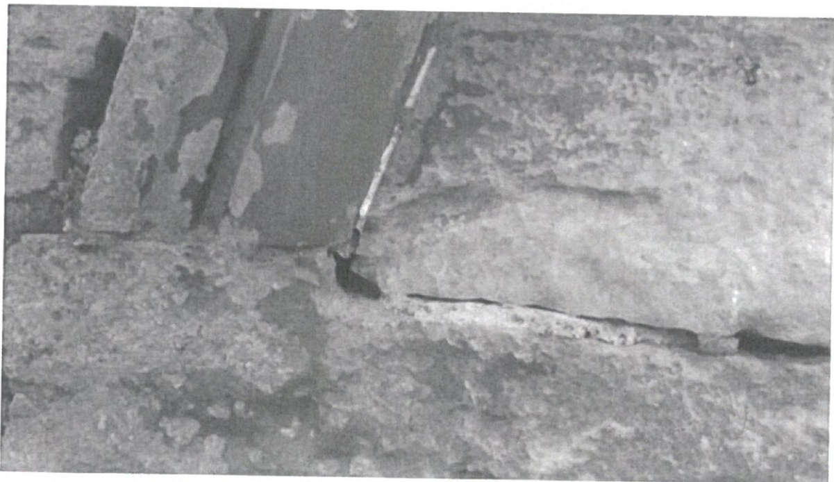
Deterioration to the mortar pointing at the apex window areas of the spire.
