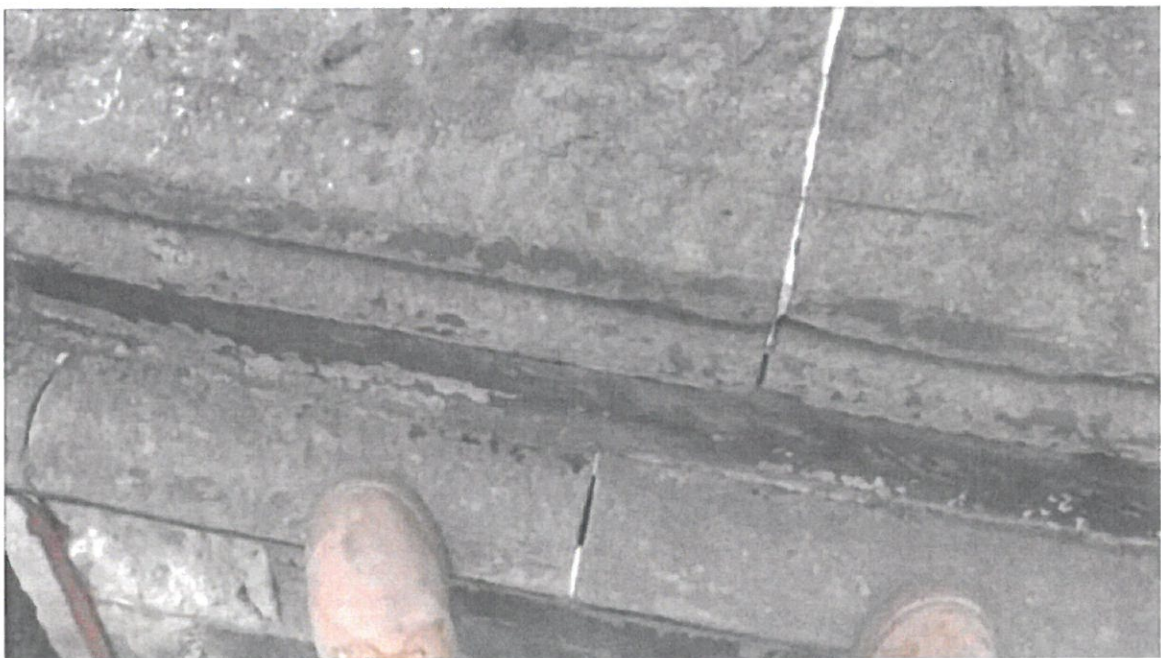
The masonry joints on the drip courses have failed in some areas.
