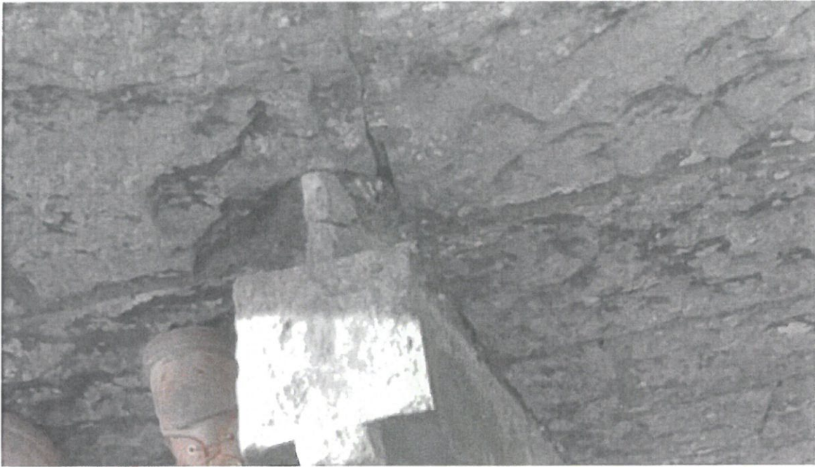
The upper stone on this pinnacle shows a section where the masonry has cracked and failed.
